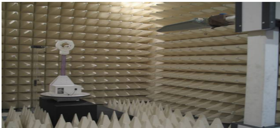
Figure2. Photograph of 3m Fully-Anechoic Chamber
