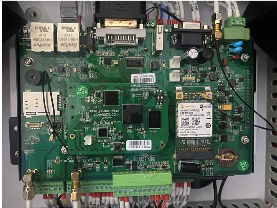
Main control board
