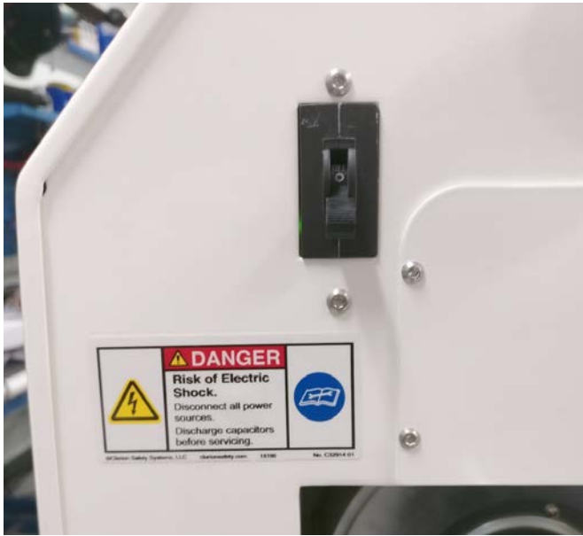
Breaker (Disconnect) Switch
