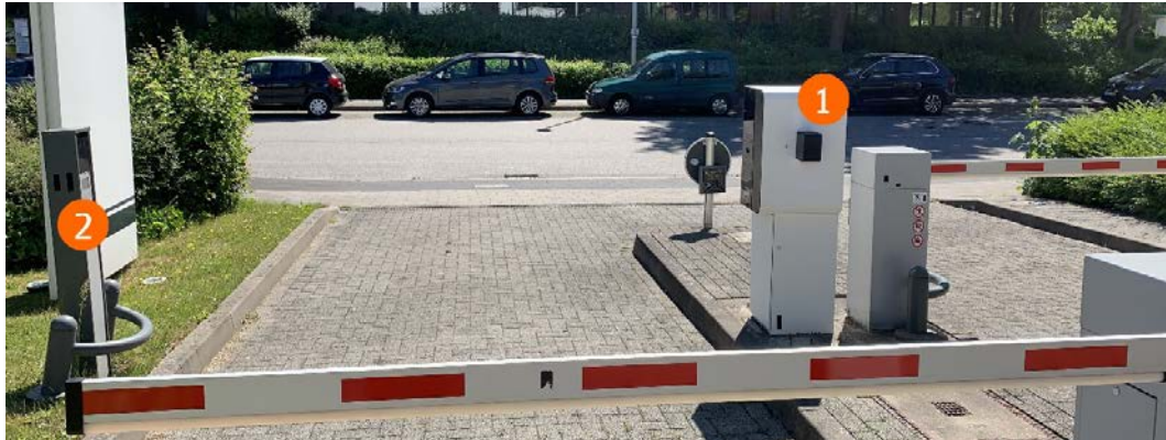
Fig. 4: Example: Installed beacons at a car park entrance
