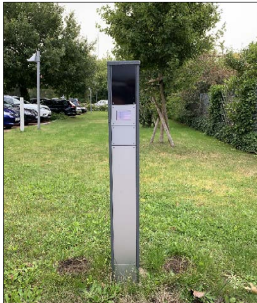
Fig. 11: Beacon in DCT casing body
