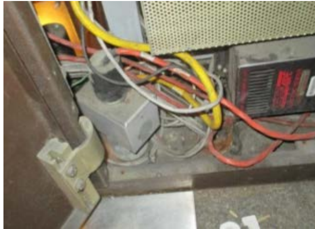
[Figure 19] Current Power Receptacle Example
