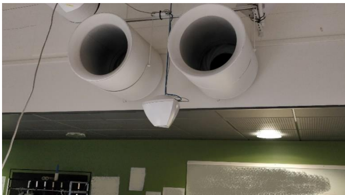
Figure 5 Part of the office has a partially lowered ceiling; therefore, the beacon is installed quite low to support also this low area
