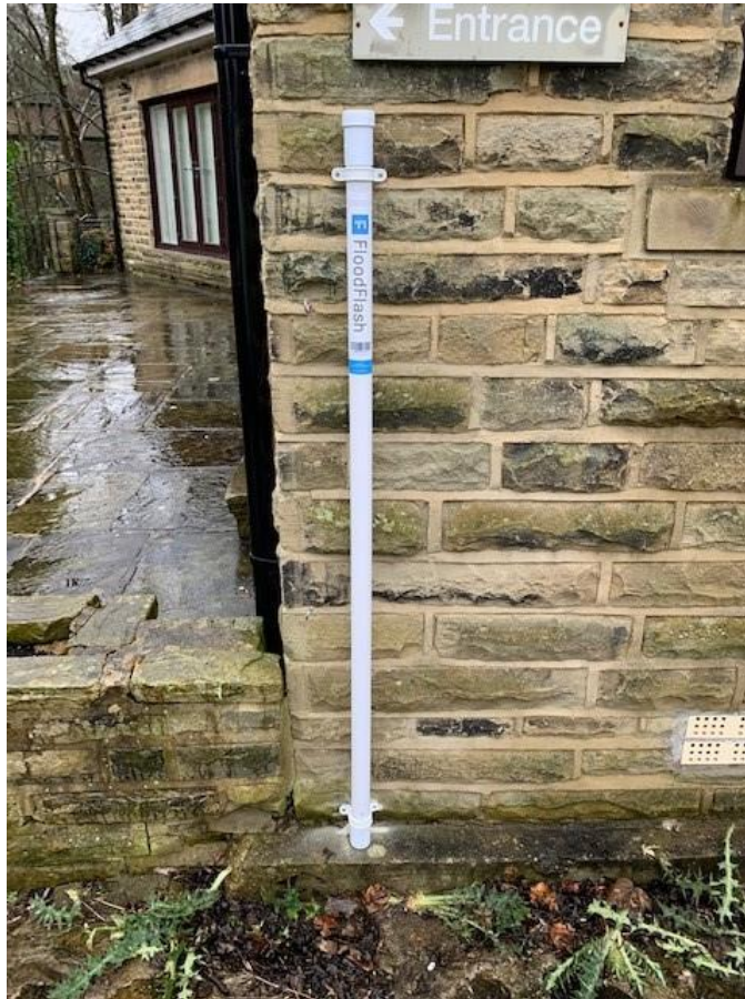
Installed FloodFlash sensor
