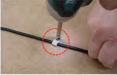
Fig.6 After fixing of control plate at table edge, organize lines with enclosed accessory and finish installation.
