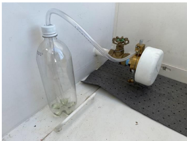
Figure 21: DGA-LT1 Ready to Bleed Air from Unit
