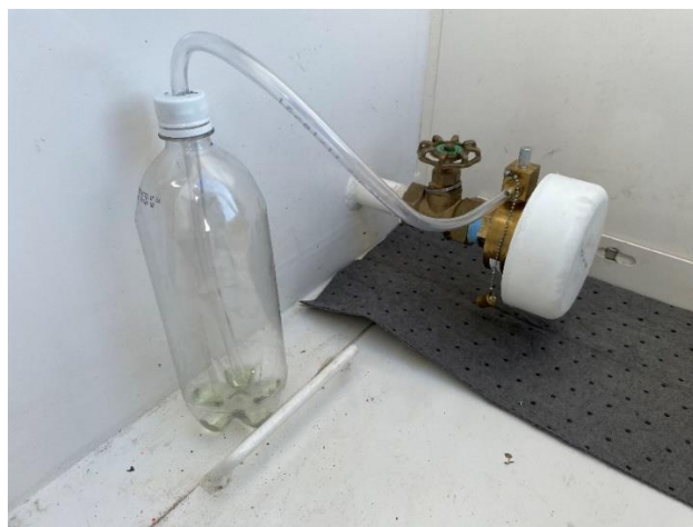
Figure 21: DGA-LT1 Ready to Bleed Air from Unit
