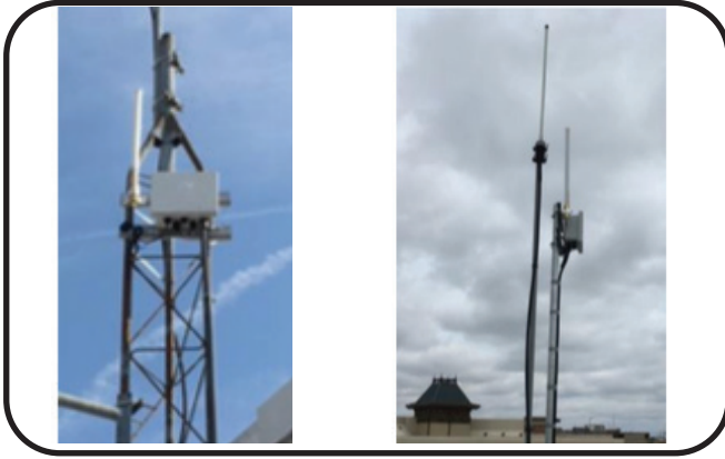
Example Roof Mount Structures
