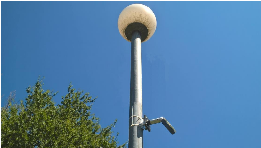
Figure 2 – HIKOB LION installed on a pole.
