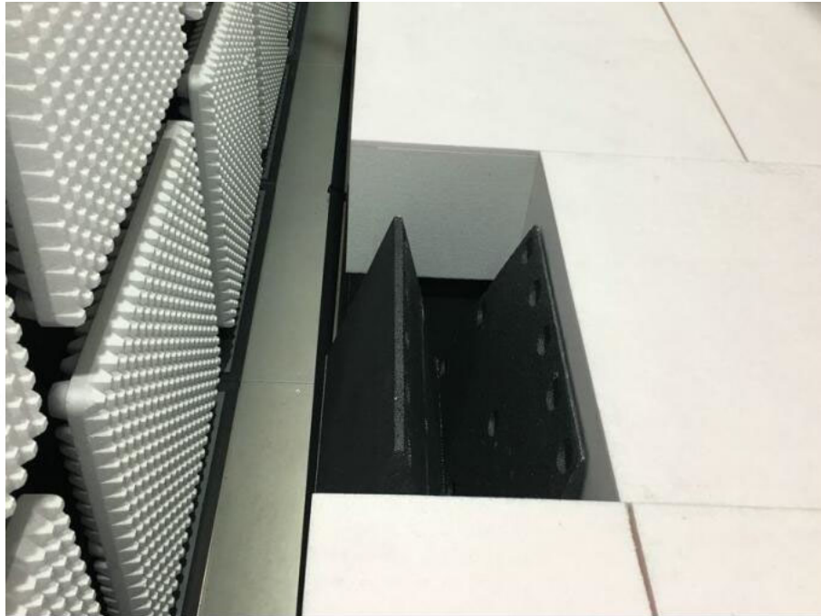
There are absorbing materials under the ground
