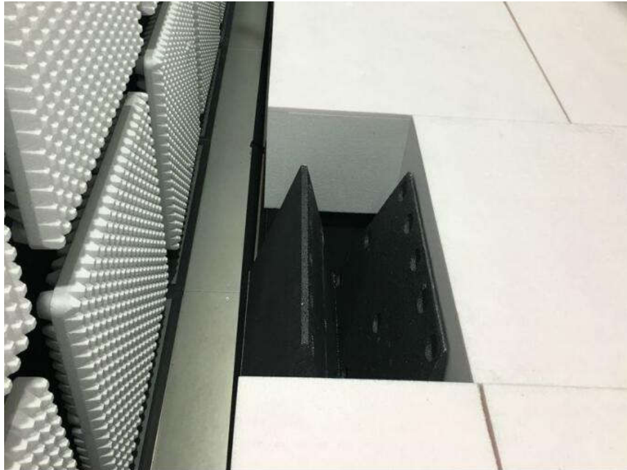
There are absorbing materials under the ground
