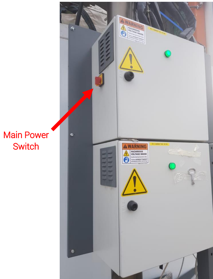
Figure 20 The Mast main power switch
