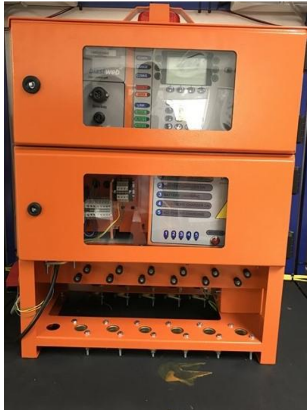
Photo 2: BCU front view
