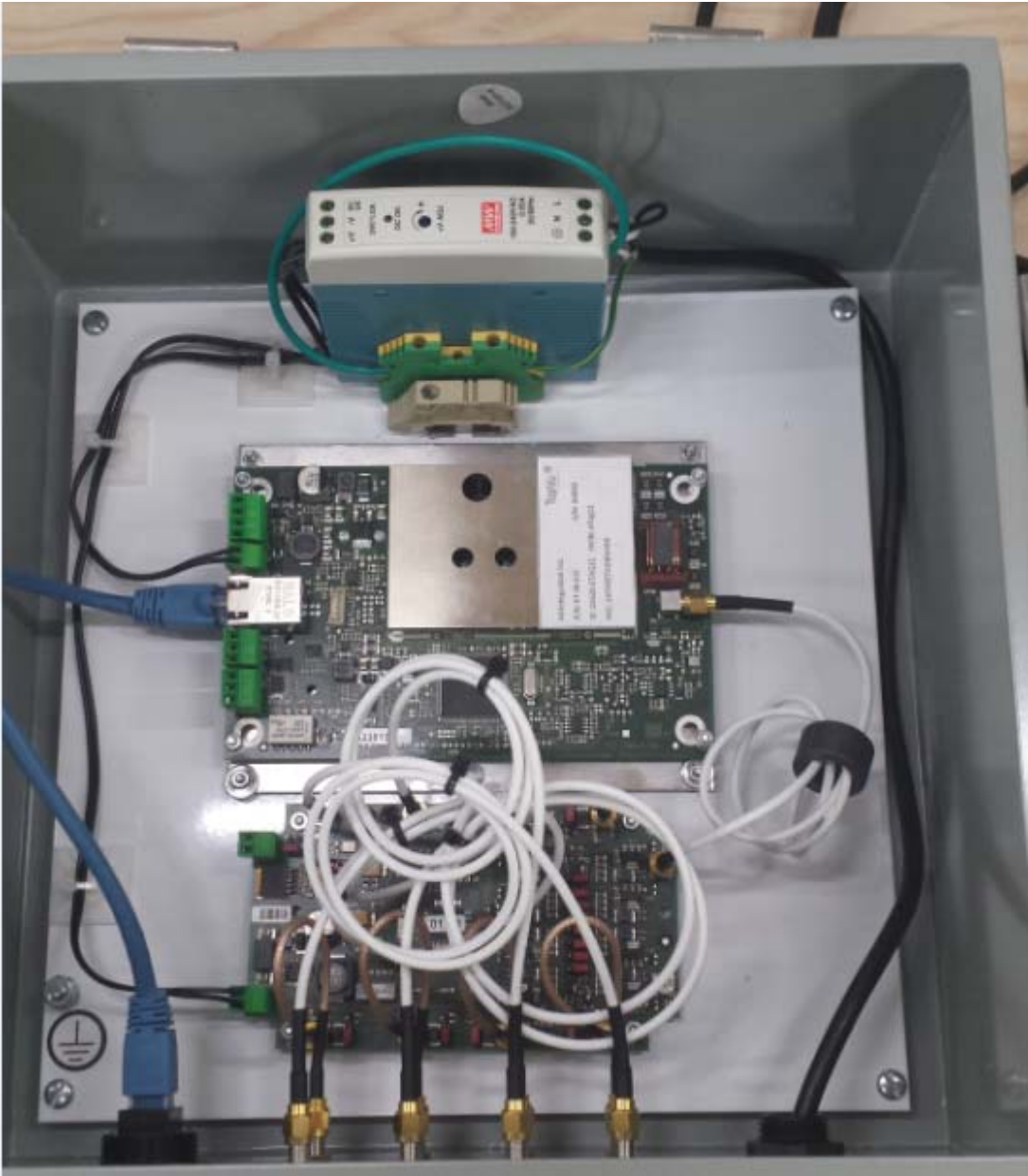
Internal Photos of the eTag ® board Control Box.
