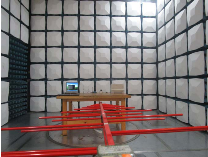
RE Below 1G Front View
