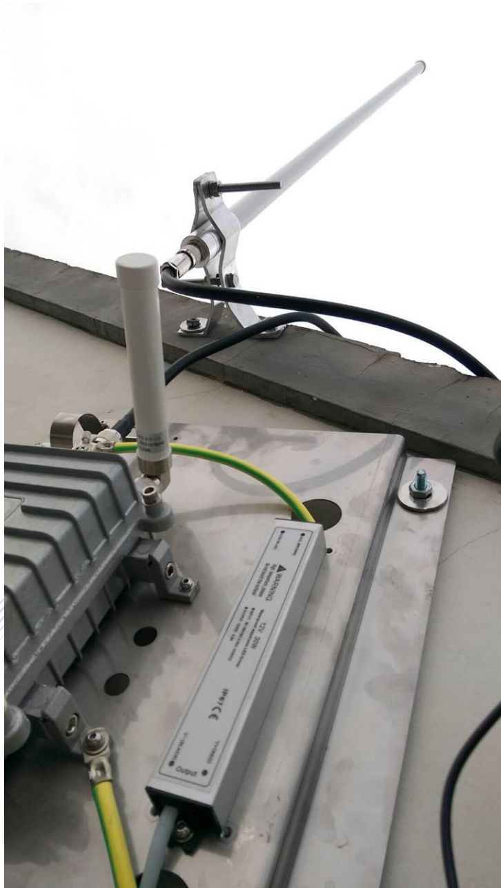
Figure 10 Antenna extension cable installation
