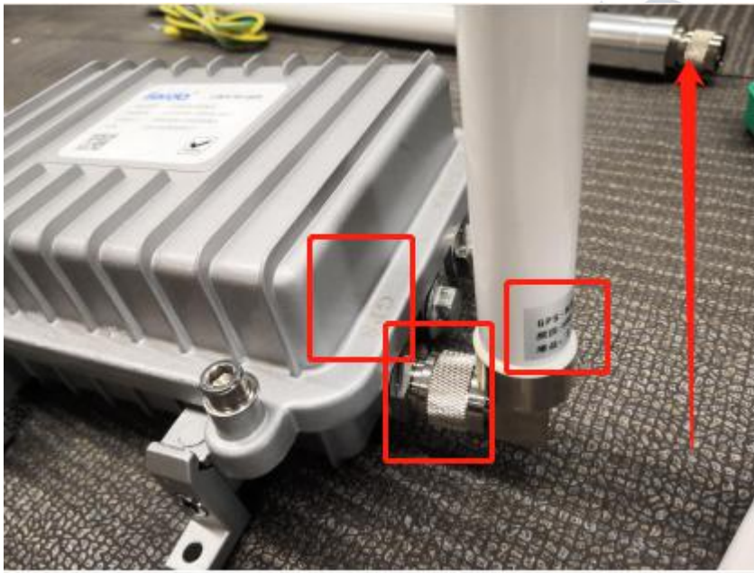
Figure 3 GPS antenna installation
