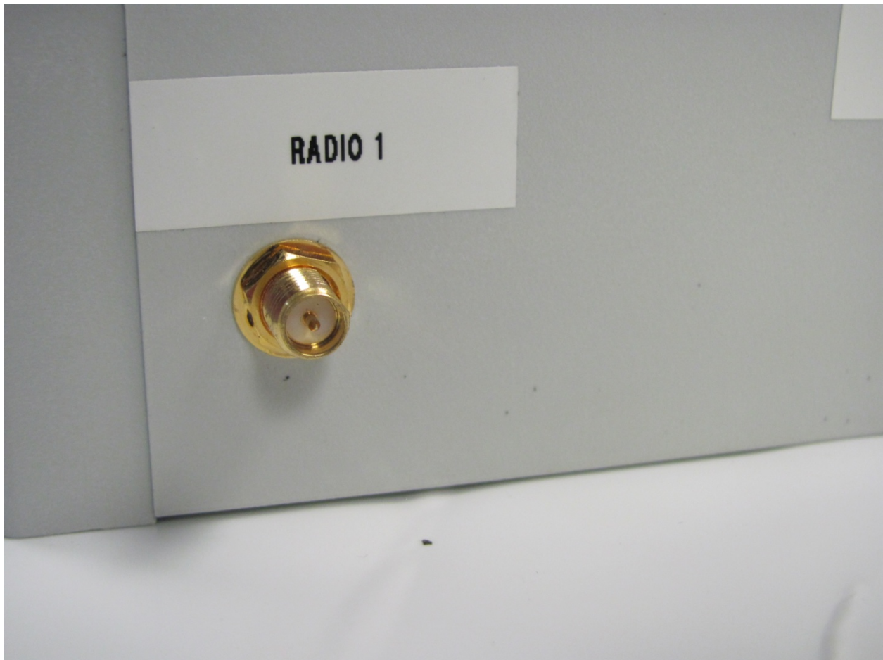
Figure 7. Antenna Port with Antenna Removed (Radio 1)
