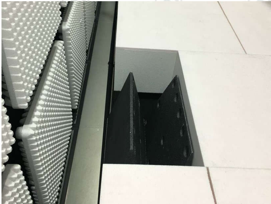
There are absorbing materials under the ground.
