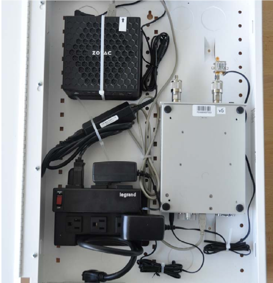
Figure 1 - Service Box Interior
