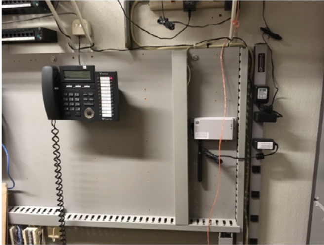
Fig.9 Metal communication board where wires come into the stockroom
