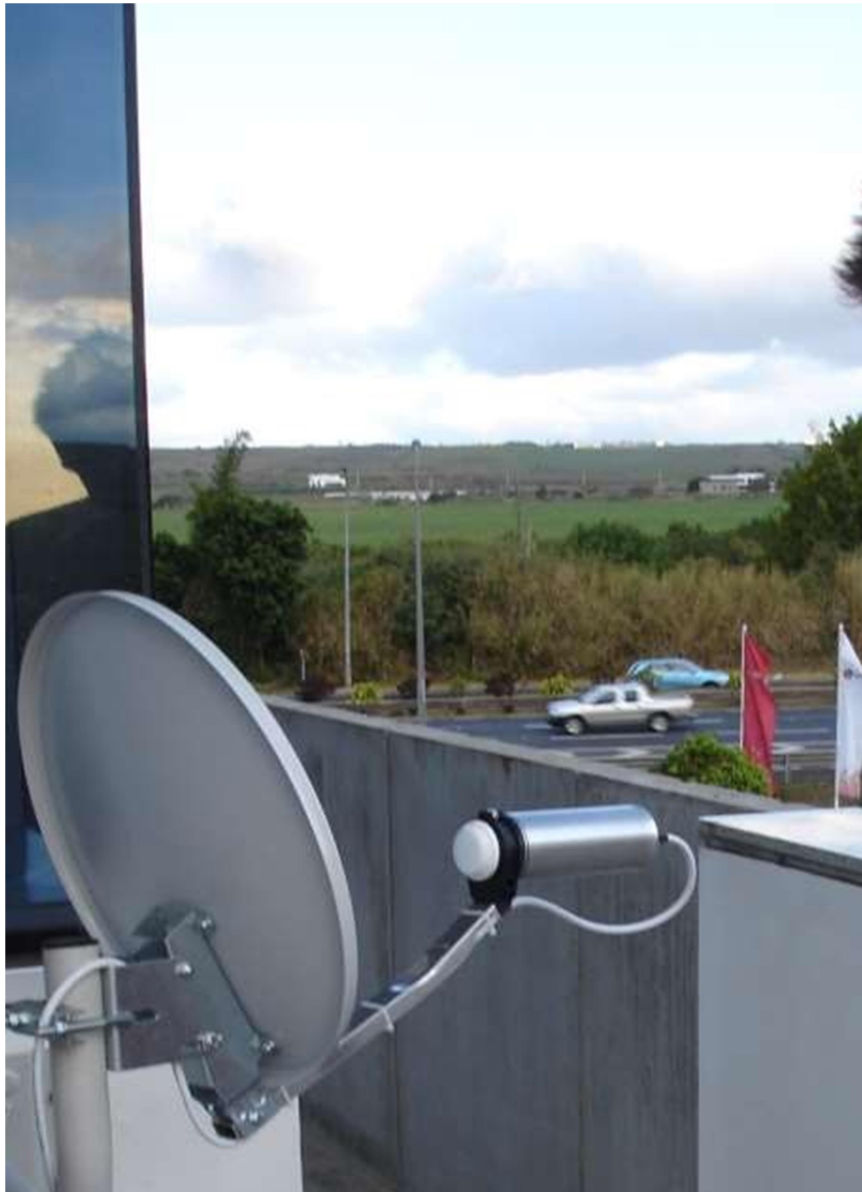
Figure 6: CASE3: unsuitable antenna site installation
