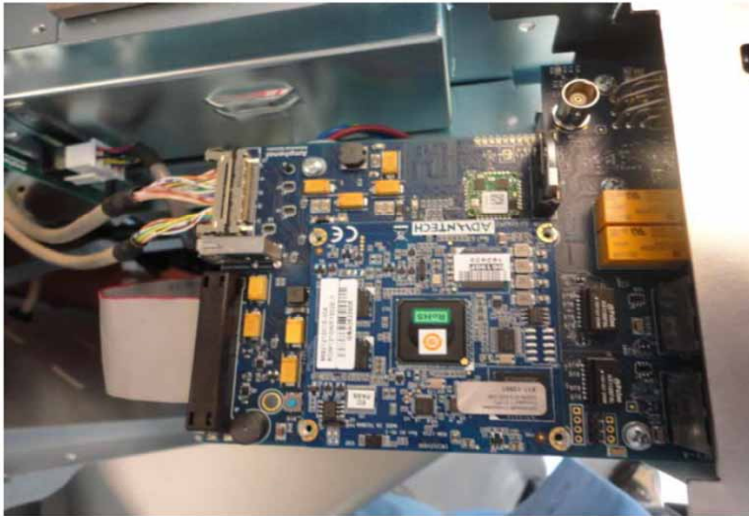
Photo 5 - Internal view of relays
