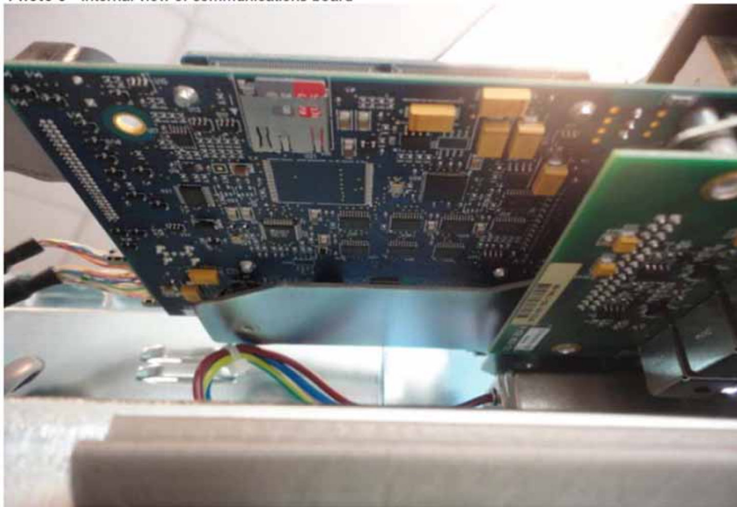
Photo 8 - Internal view of communications board
