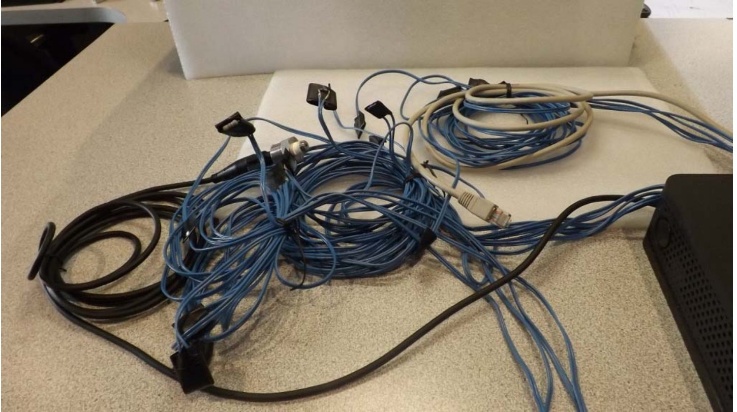
Figure E23.9 – Setup – Cable Terminations
