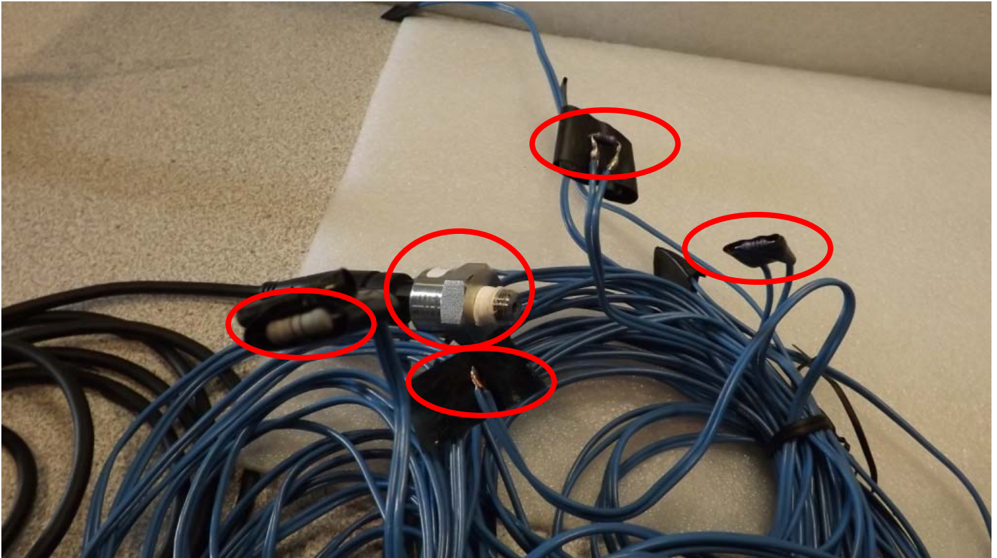
Figure E23.10 – Setup – Cable Terminations
