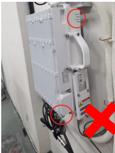
The RF feed system does not connect, the cell is activated and RF transmits signal
