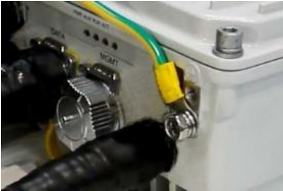
Figure 4-17 Connect GPS Lightning Arrestor Grounding Cable
