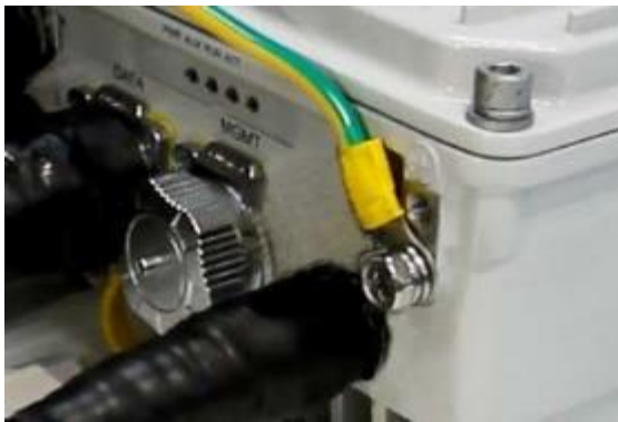
Figure 4-17 Connect GPS Lightning Arrestor Grounding Cable
