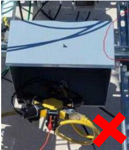
Disordered wiring of distribution box
