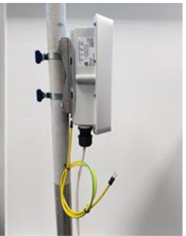
Installation the Wirnet™ iStation on the support
