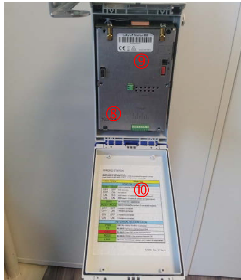
Figure 5 : LoRa IoT Station casing - internal view
