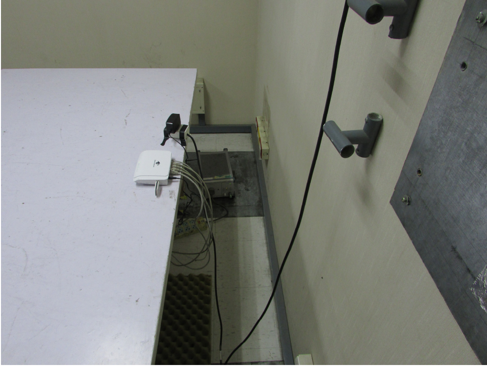
Description : Back View of Conducted Test
