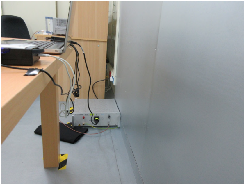
Photograph 8: Set-up for AC Mains (Back View)
