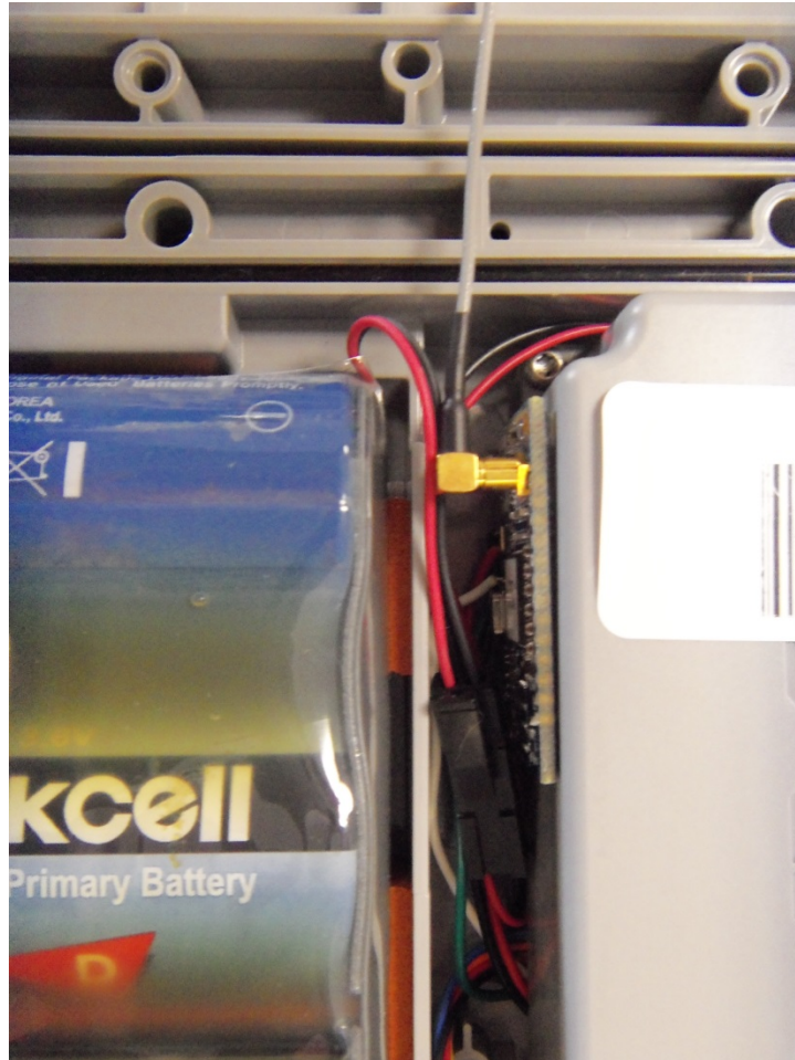
Enclosure Open, showing connection to 2.4 GHz Transceiver
