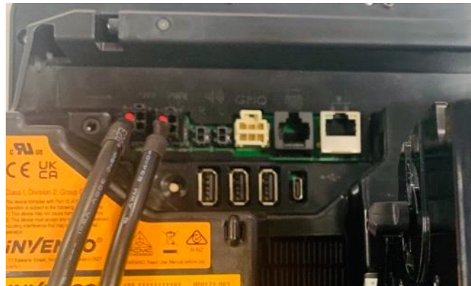
Fig. 12.3: Low-voltage DC cables
