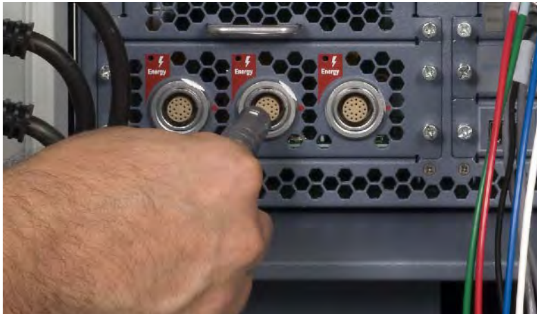
Figure 4.14 Auxiliary device connections (back of Core)
