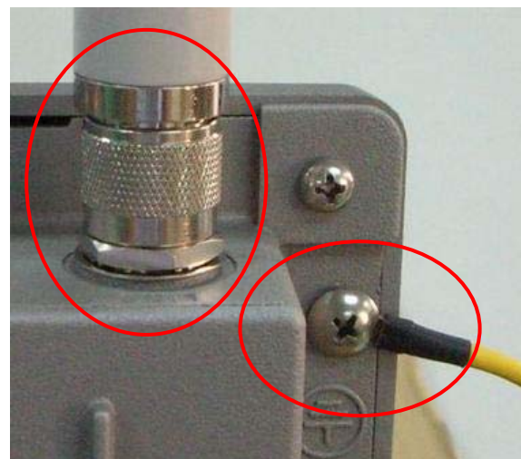
Figure 7 – secure antenna and grounding cable
