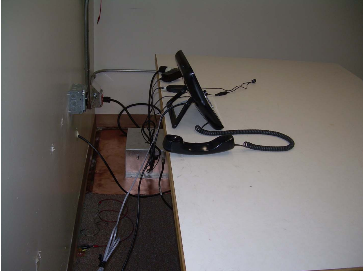
Photograph 4 – Back View Conducted Disturbance Worst Case Configuration
