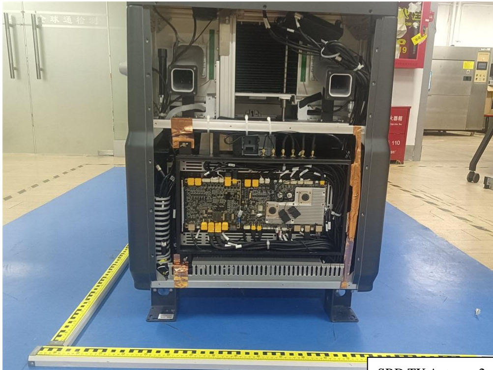
SRD TX Antenna 2
