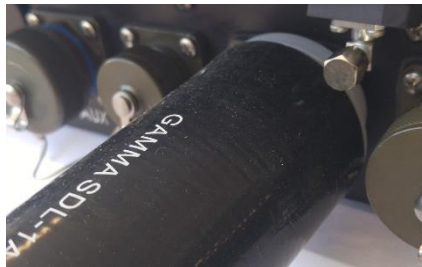
Figure 11: Cold Shrink Bulkhead Placement
