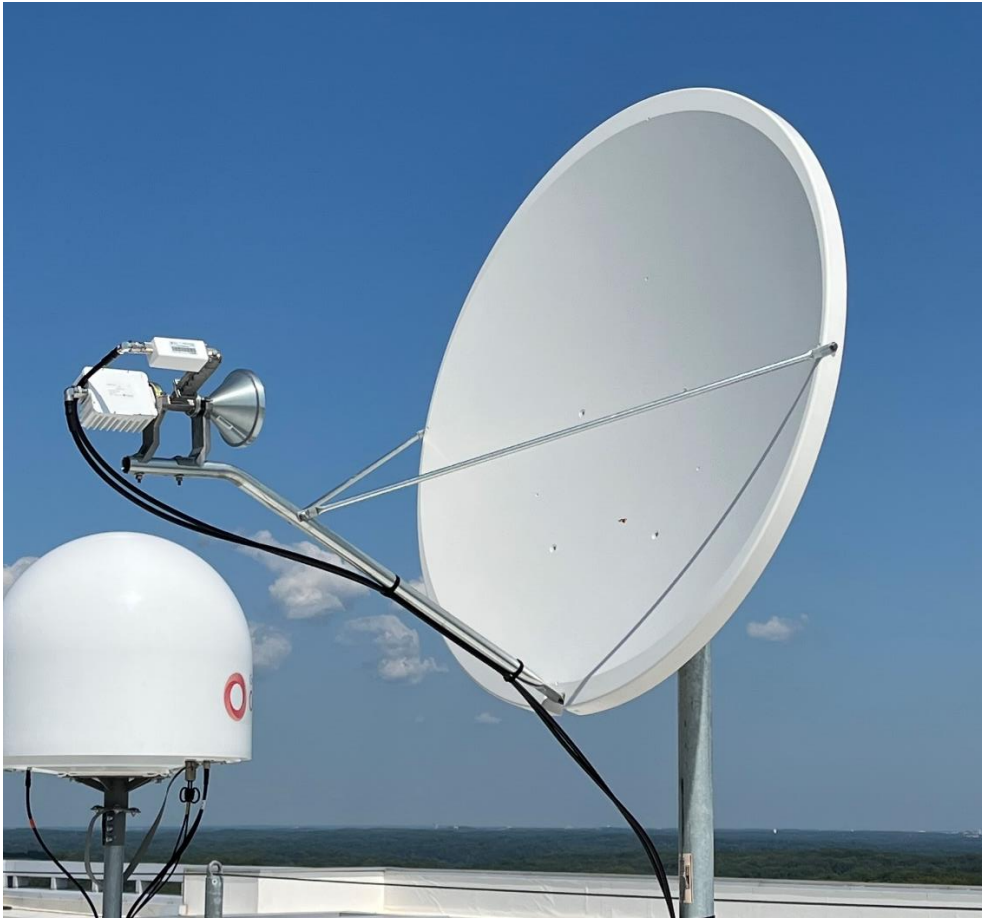
Figure 2. CPI Prodelin 1132 Dish placed atop MITRE at N 38 55 24, W 77 12 21
