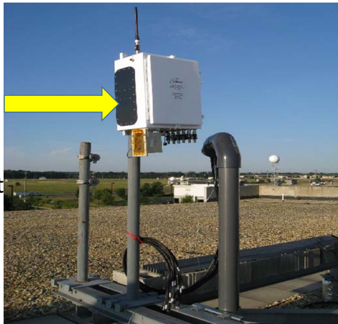
Figure 1 Photo of Tampa Microwave Emulator Installation
