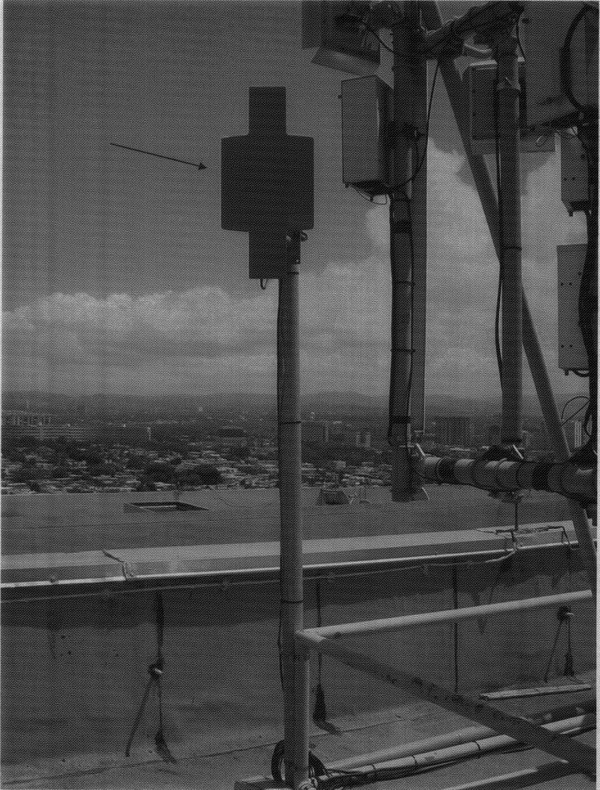
Figure 7 – Mast #2 with NEP5 emitter.
