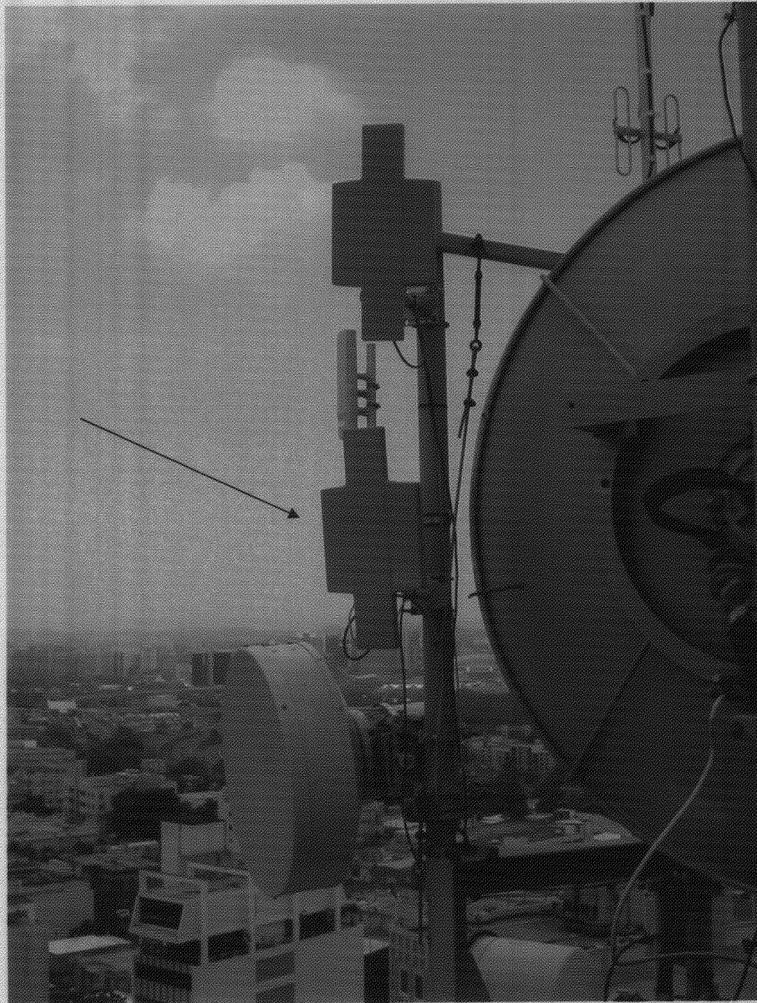
Figure 4 – Mast #1, Antenna 1 (bottom).
