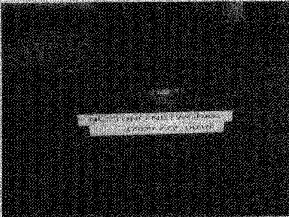
Photo 4 – Neptuno Networks cabinet at Site 3 Cerro Pina
