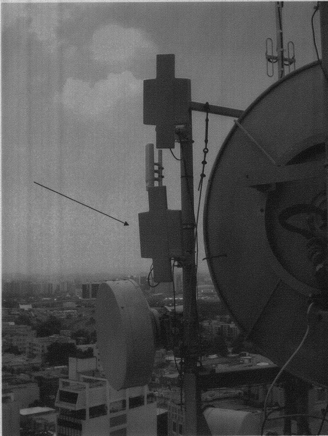
Figure 4 – Mast #1, Antenna 1 (bottom).
