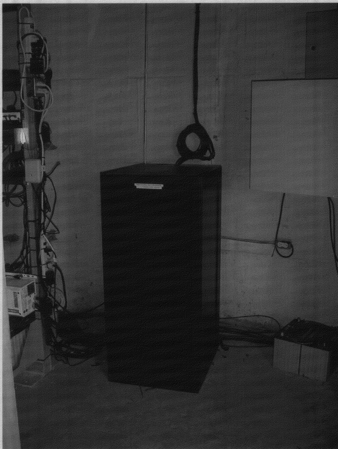
Figure 11 – Neptuneo equipment cabinet.
