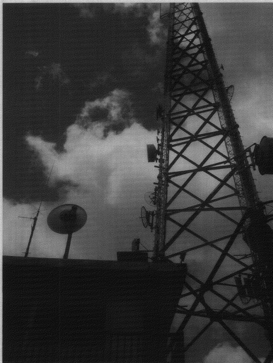
Photo 6 Apparent Neptuno Networks Antennas (between two upper microwave dishes) at Site 4 Gurabo
