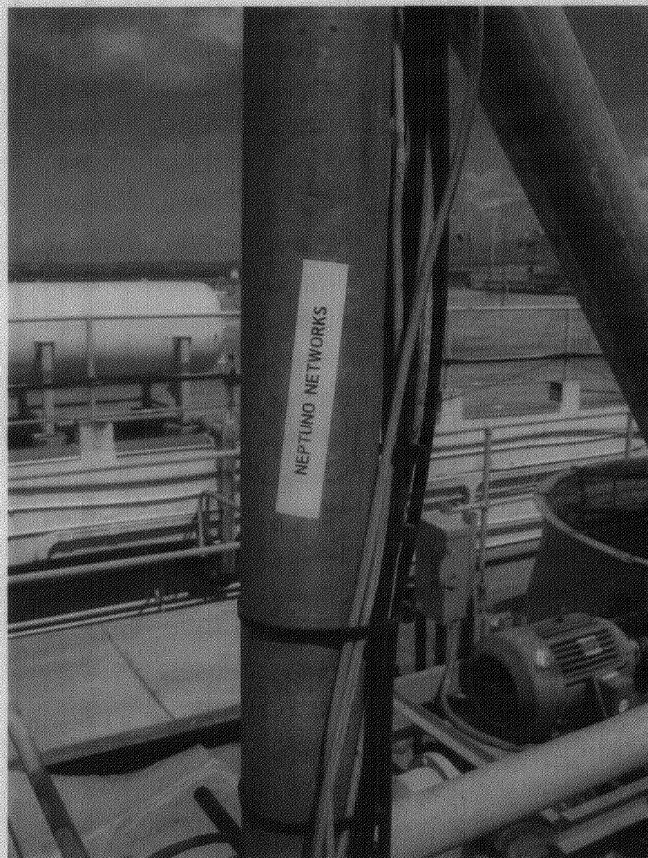
Photo 2 – Neptuno Networks ID on Mast shown in Photo 1
