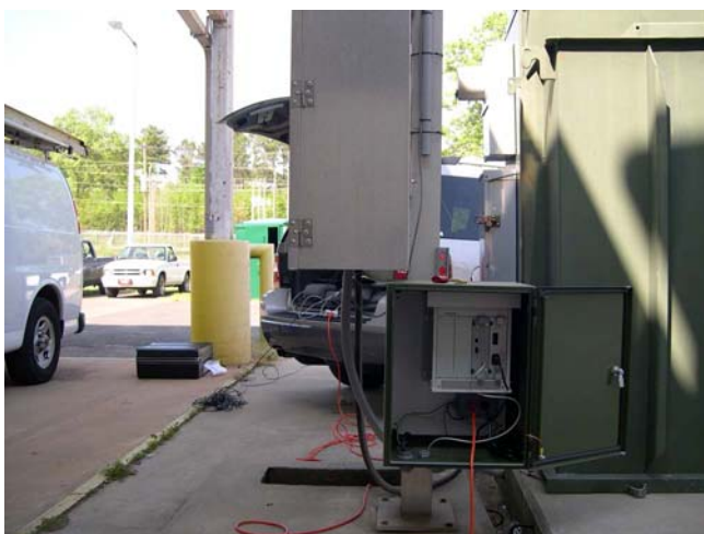
JEMC Location - Pad Mount Transformer
