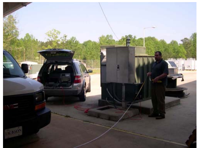
JEMC Location - Pad Mount Transformer
