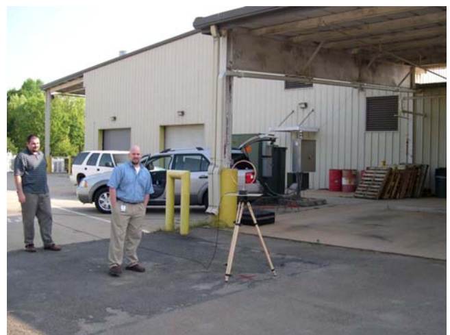
JEMC Location - Pad Mount Transformer
